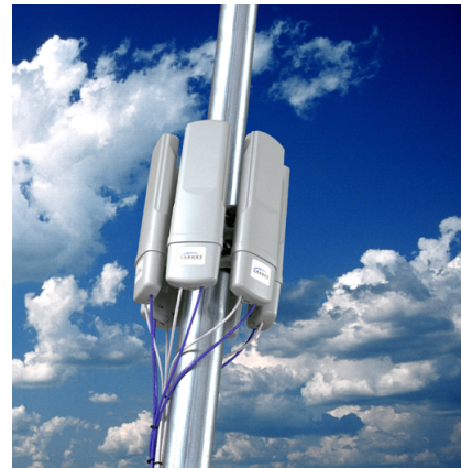
Figure 1: Pole-mounted AP cluster
